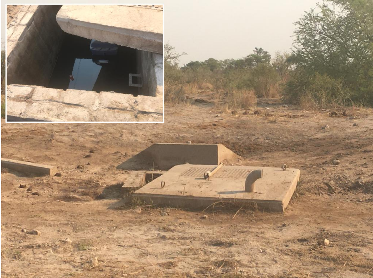
Figure 21: Evidence of elephant accessing water from the pipeline to Phuduhudu village
